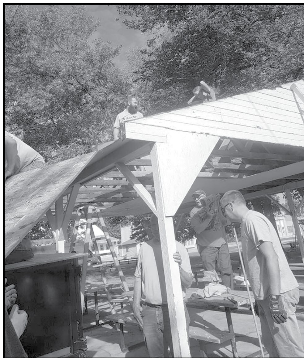
Volunteers worked on making improvements to the Carroll Park over the Labor Day weekend. Above, volunteers replaced the roof of the park's picnic shelter.
